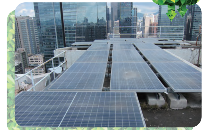
Solar panels installed in Laguna City, one of our Managed Properties
