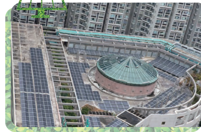
Solar panels installed in Laguna Plaza, one of our Managed Properties
