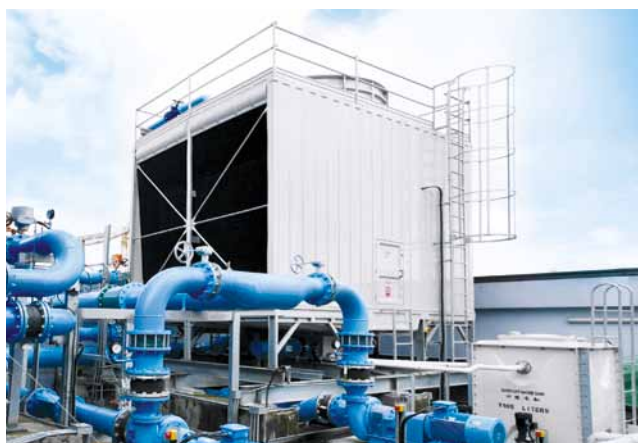
Water-cooled air-conditioning system at 248 Queen's Road East
