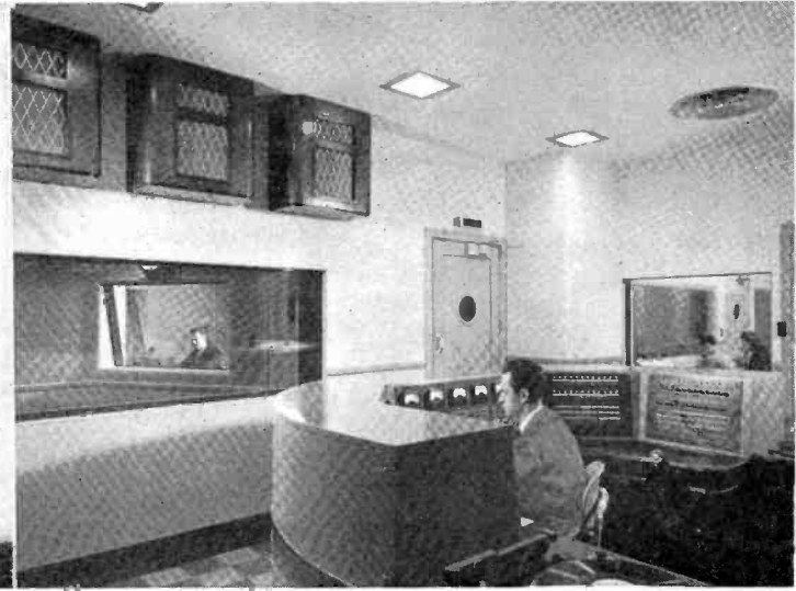
MASTER CONTROL ROOM, center of technical operations. It handles switching functions of six studios. Operator can see into three studios.
