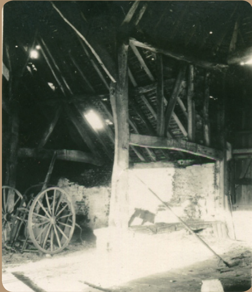
View of barn interior: 1948. Note intact roof. (Reproduced by permission of Les Bowerman).
