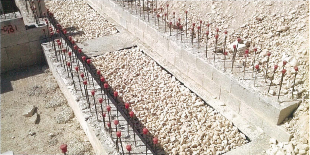
Clean gravel in two of the planter pits. GHRC.
