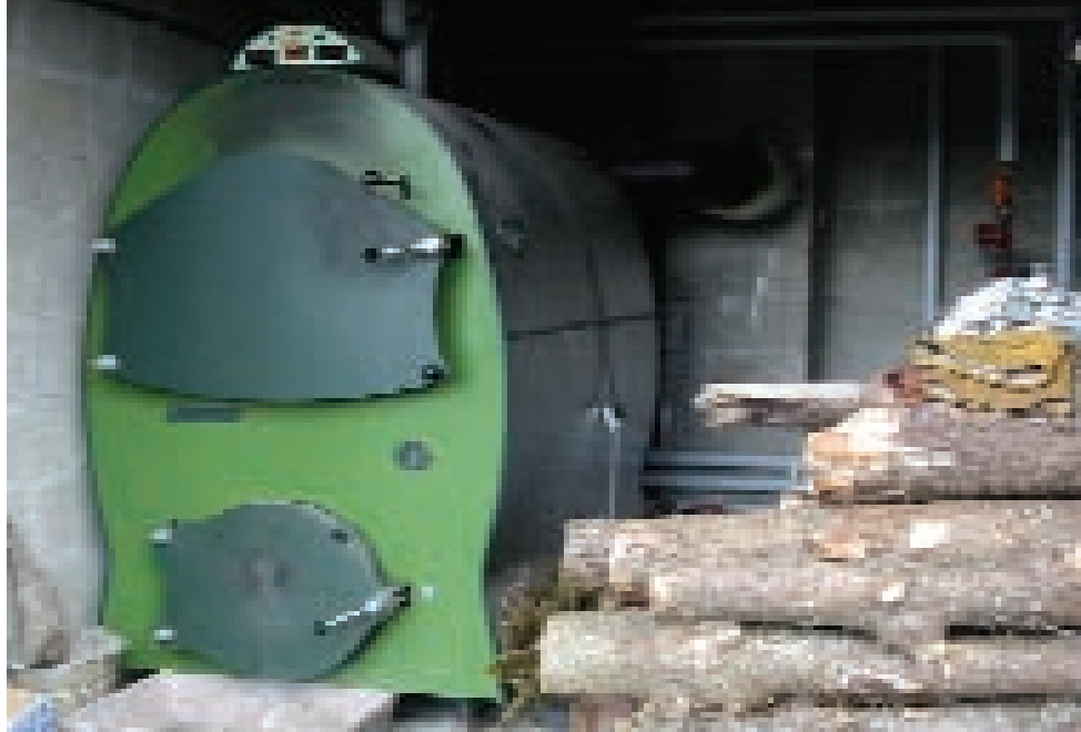
The Sustainable Land Use Company's log boiler
