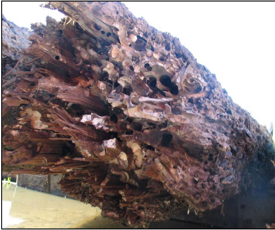
Figure 14 Severely infested pile from pier 4
