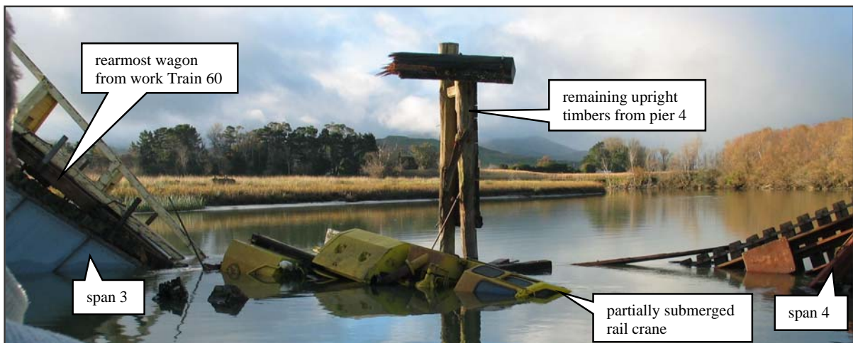
Figure 1 Bridge 256 following the collapse
