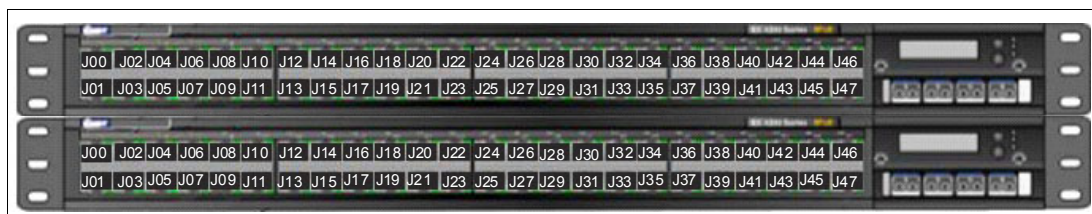
Figure 7-8 Two 1000BASE-T TOR switches (INMN)
