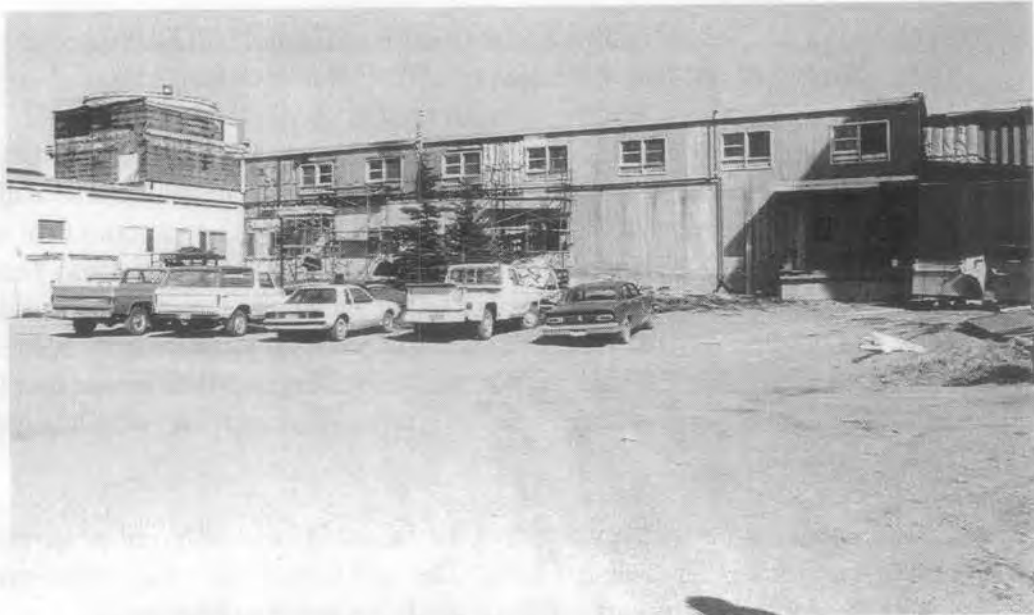
The control building at Nike Site Bay being remodeled for use as a correctional center.
