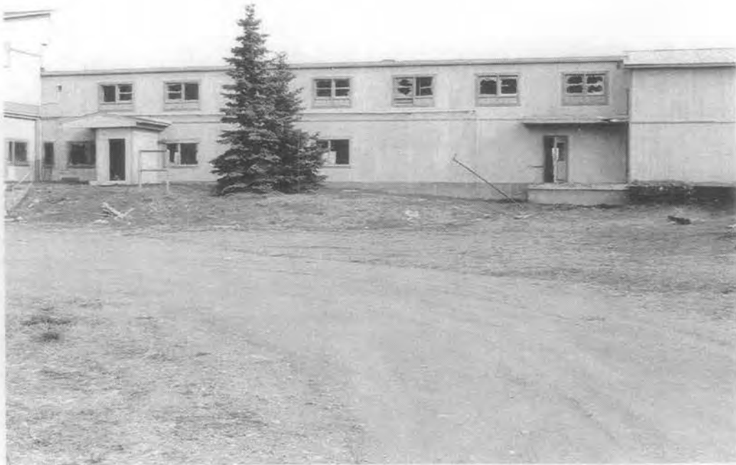
Another view of the vandalized correctional center at Nike Site Bay.
