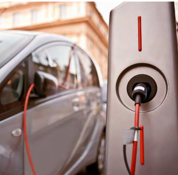
Electric car charging station.
