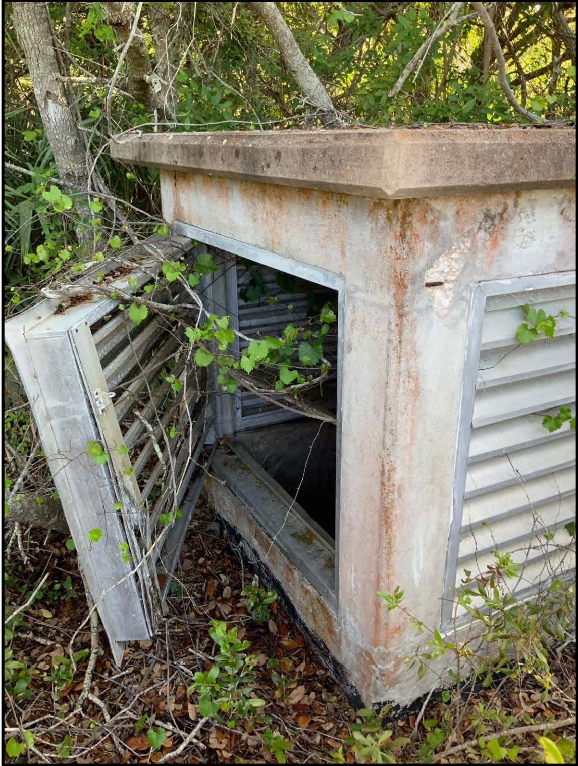
Figure 8. Vented structure attached to a tunnel located in LMU 18 - view facing S.
