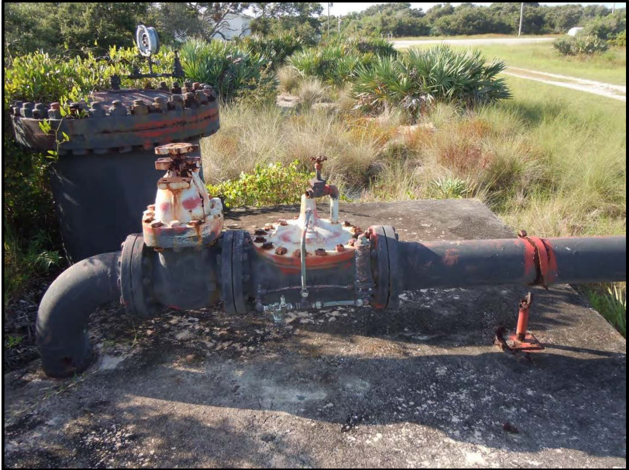
Figure 7. View of water pump on structure preliminarily identified as a Thrust Block and Valve Pit - view facing S.
