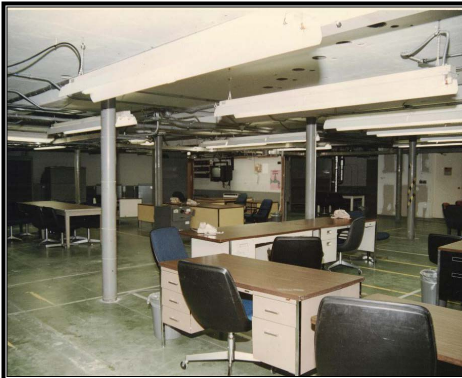
Figure 72. Photograph of the first floor office area during its use in 1993 (Bionetics Corp. 1993c).
