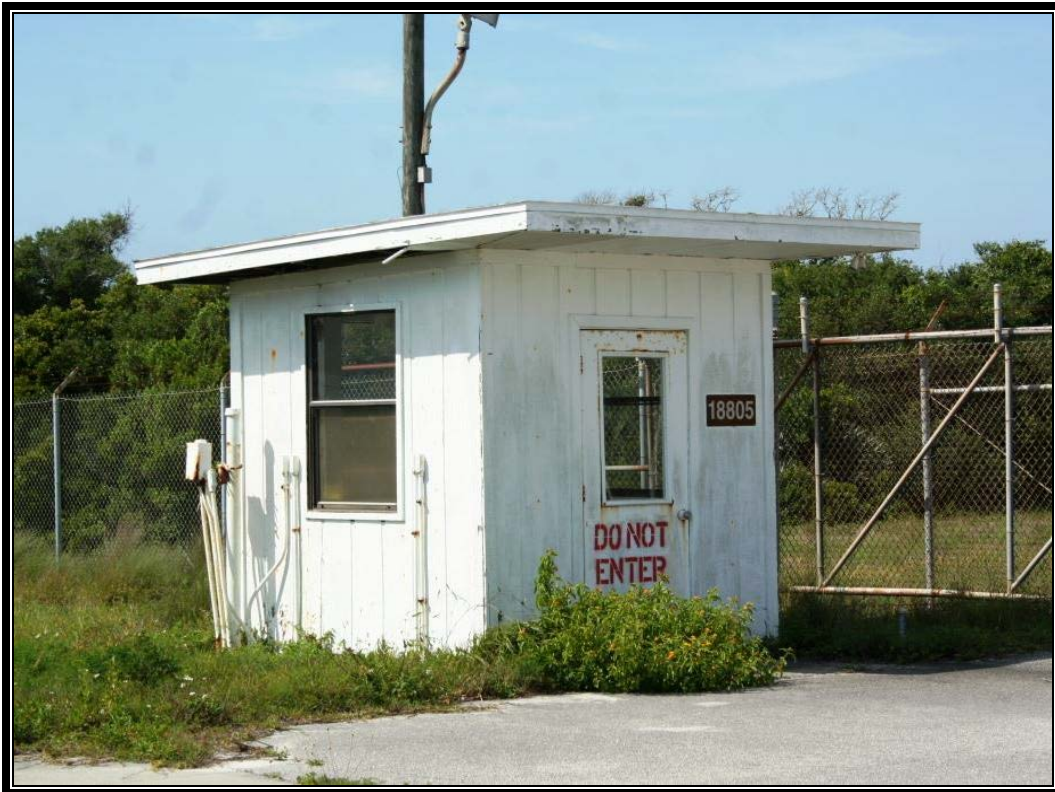
Figure 76. View to the southwest of Facility 18803 (note incorrect facility number on bldg).
