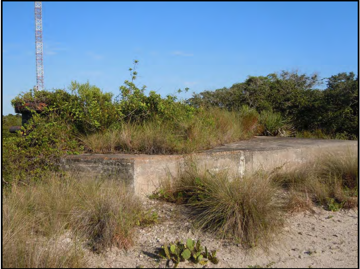
Figure 6. Backside of structure preliminarily identified as a Thrust Block and Valve Pit – view facing W.
