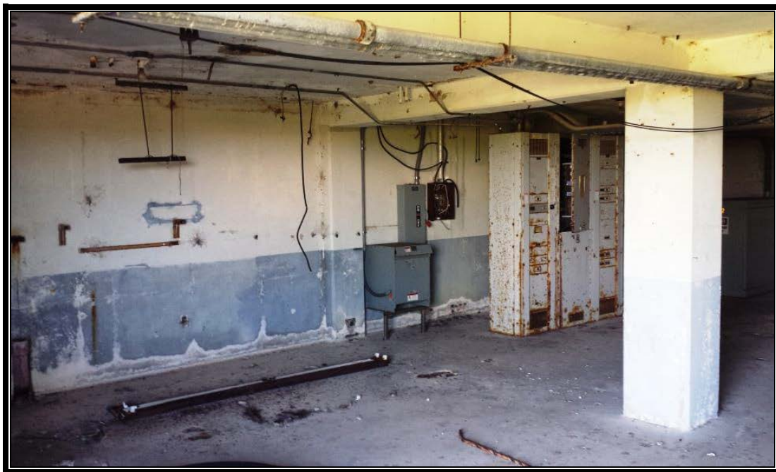
Figure 46. Interior photograph of Facility 15500B showing current conditions and electrical components from the Red Tigress program.
