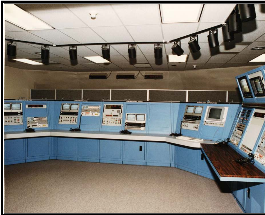
Figure 71. Photograph of the launch control center during its use in 1993 (Bionetics Corp. 1993b).
