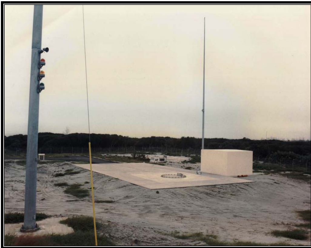
Figure 57. Photograph from 1989 showing Facility 15640-Launch Pad B-BMDO under construction (Bionetics Corp. 1989b).
