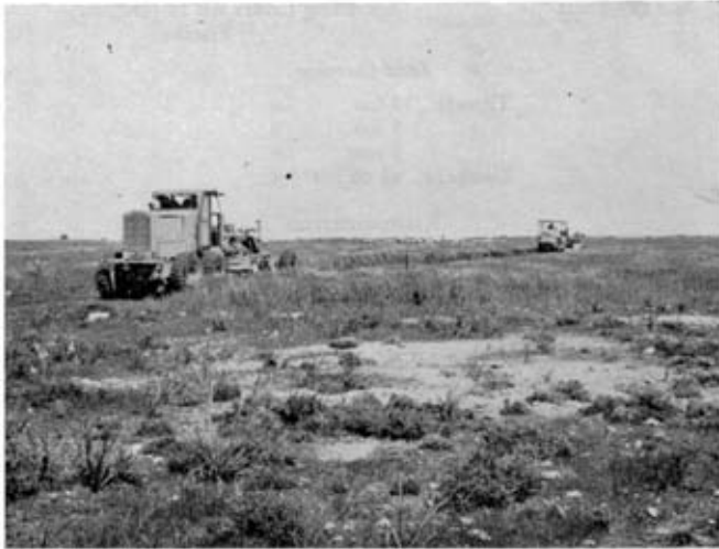
Photo 1. The D8H leads a grader through the barley to "prove" our right to build the airstrip. A small area of caprock can be seen in the foreground.
