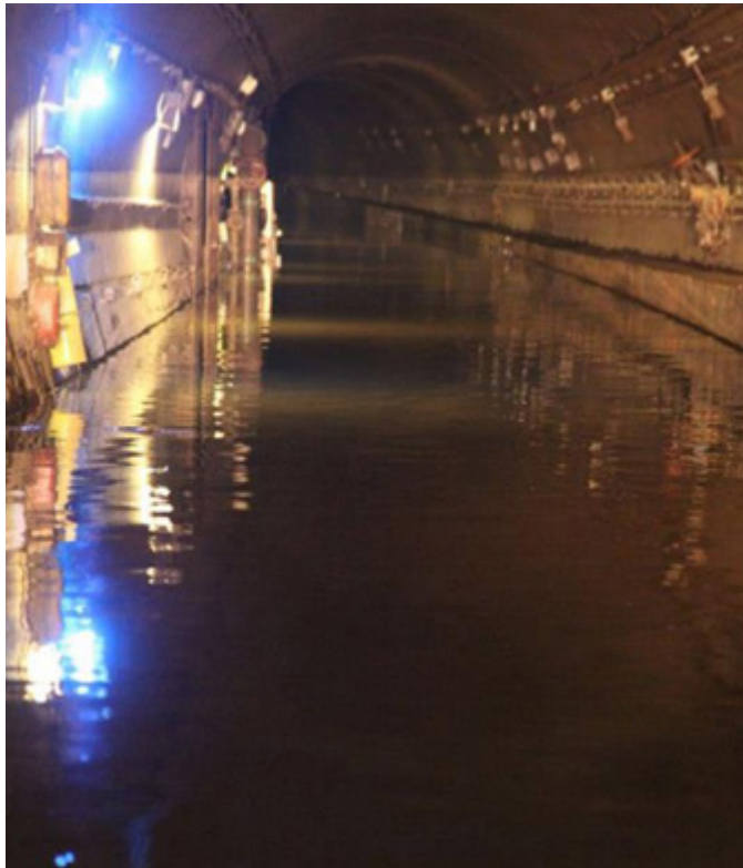
FLOODED SUBWAY TUNNEL FROM HURRICANE SANDY
