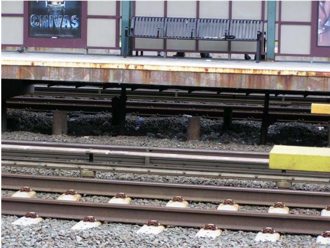
Figure 2. Center platform under which passenger crawled, crossing into path of oncoming train.
