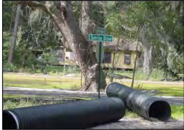
The sewer comes to Sunrise Drive in the Harrington section of St. Simons Island, GA. For sale signs soon followed.
