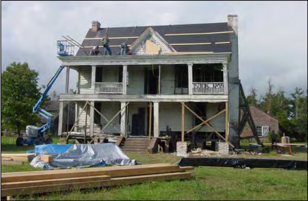
In 2002, the house at Tibwin was stabilized and re-roofed by the NPS Williamsport Preservation Center.
