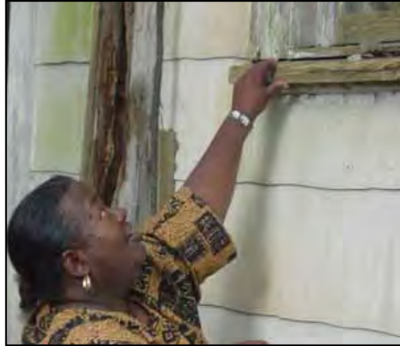
Amy Roberts examines deteriorating window sill, Harrington School House. SSAAHC hopes to restore the school as a museum or community center on St. Simons Island, GA.
