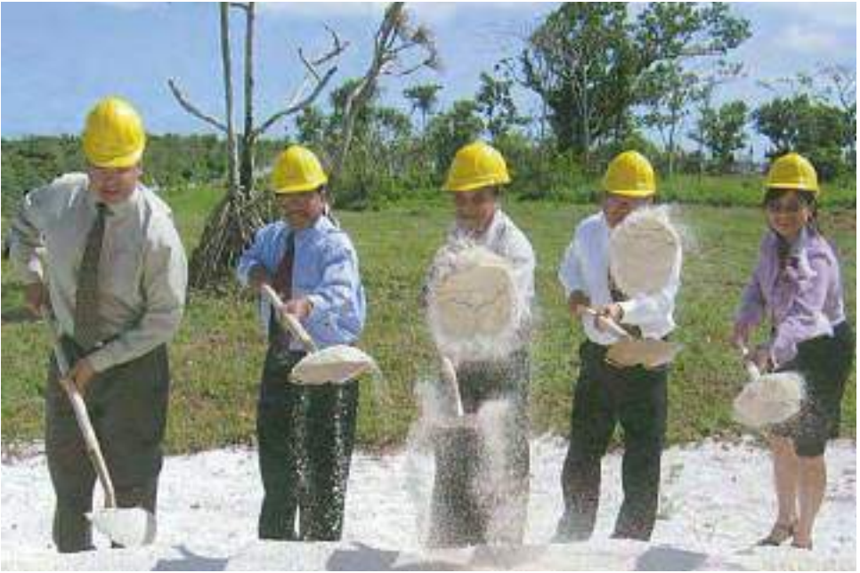
Groundbreaking for the Rota Judicial Center (January 2004). Left to Right: Associate Justice John A. Manglona, Associate Justice Alexandro C. Castro, Mayor of Rota Benjamin T. Manglona, Chief Justice Miguel S. Demapan, Judge Ramona V. Manglona.
