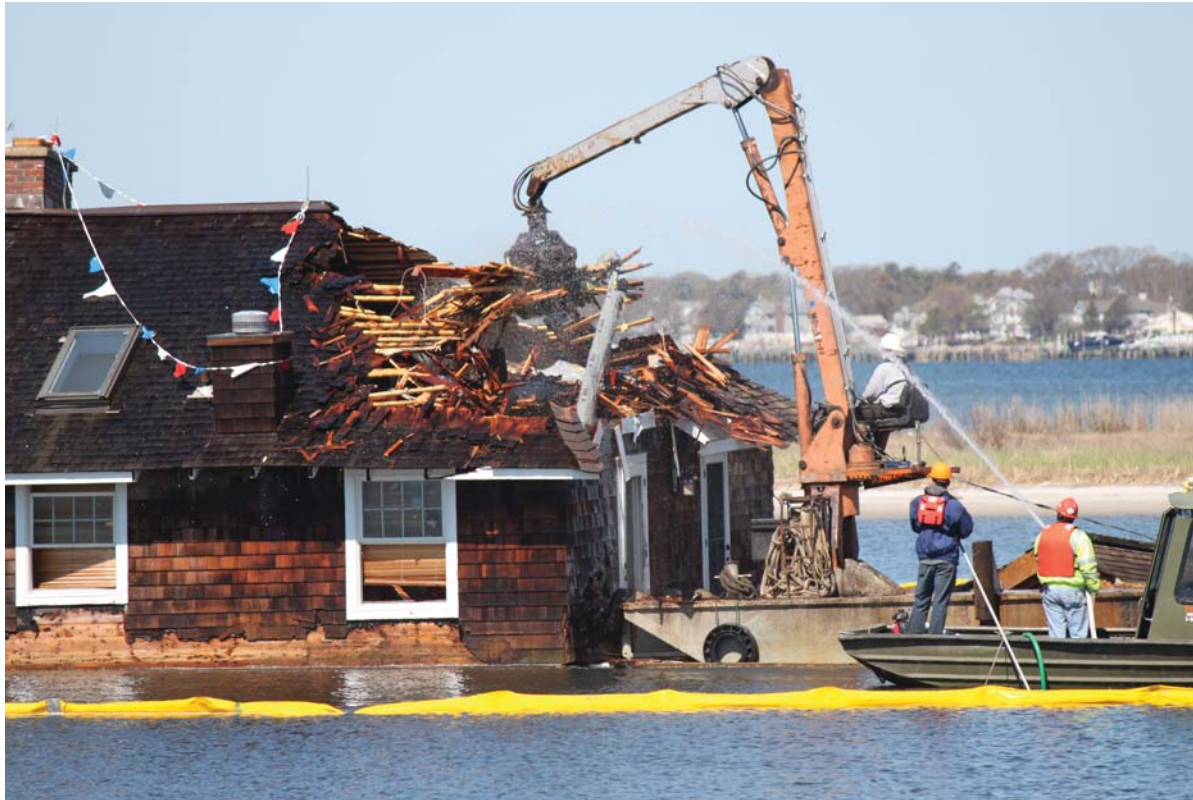
Post-Sandy debris removal.
