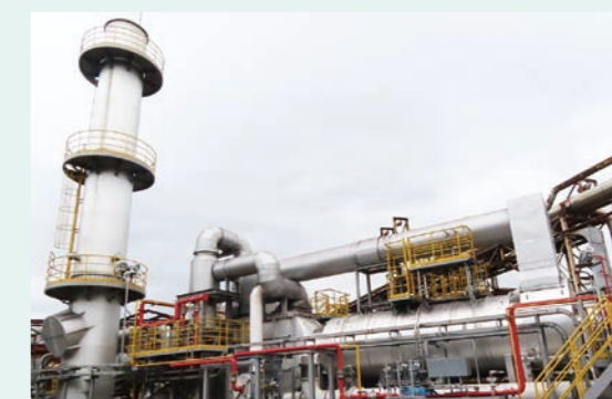
Exhaust gas burning furnace in the East Nippon Works Kimitsu Area
