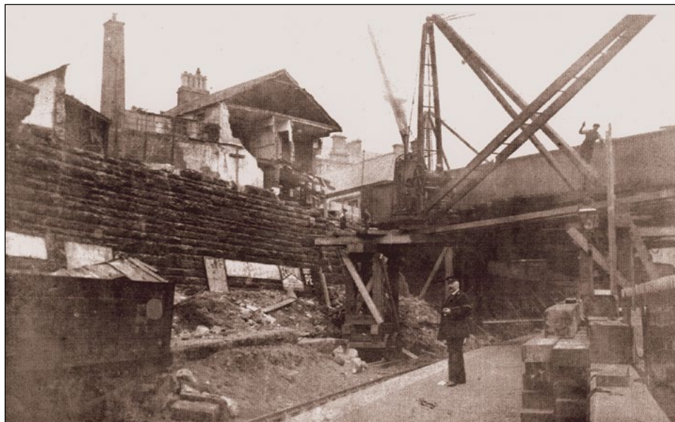
Repair work under way on the damaged wall and shop. Note the gantry construction used to keep the crane clear of the trains, which would still be running while the work was in progress.
