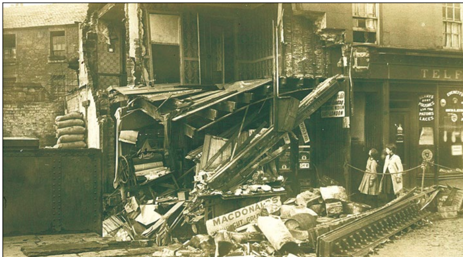
Miss Marshall's Book and stationers shop at No.27 Inverkip Street after the gable wall had collapsed. The upper floors, which comprised residential dwellings, were later removed.
