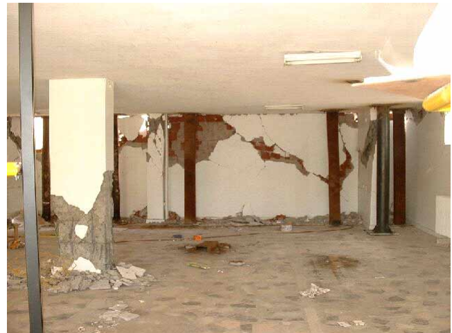
Fig. 9 Shear failure in a column partly due to inadequate reinforcement
