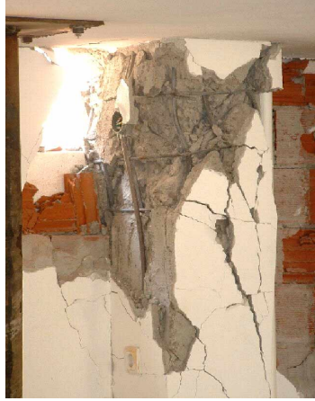
Fig. 10 Short column effect resulting in explosive shear failure
