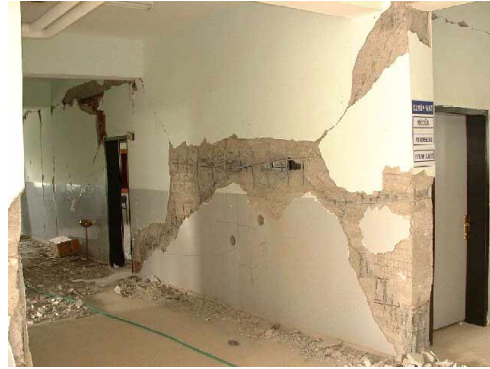
Fig. 13 Damage to the shear wall at Bingol Lisesi
