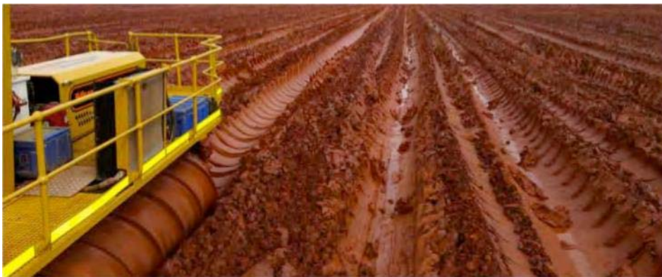
Fig. 3.18 Amphirol operating on a tailings beach showing swale drains being formed (photo courtesy of, D. Brett)
