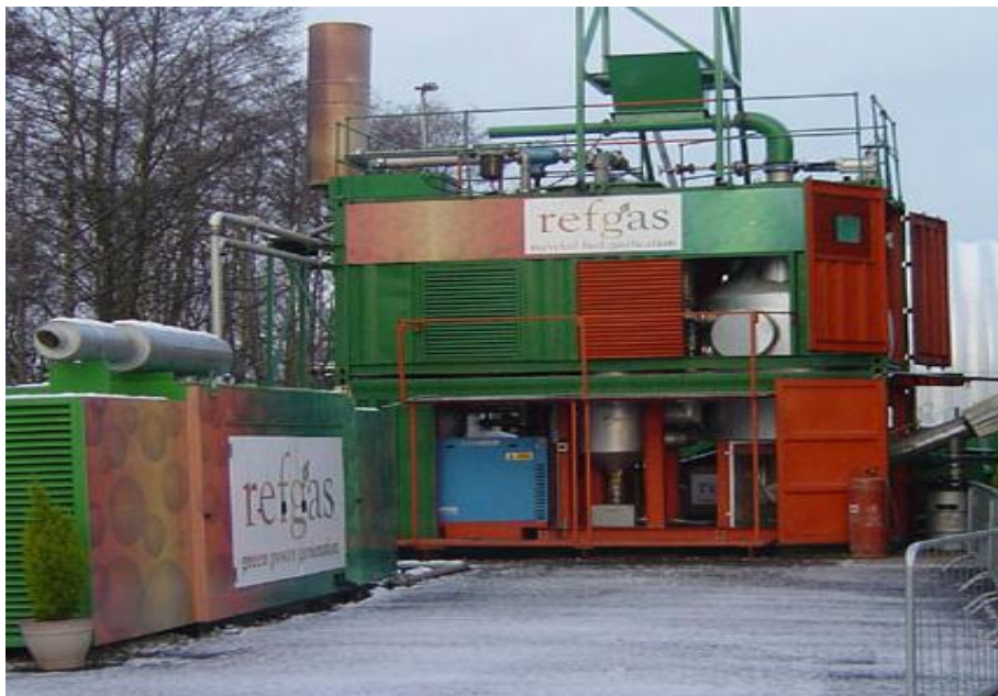
Figure 5 – photograph of a small-scale Advanced Thermal Technology facility
