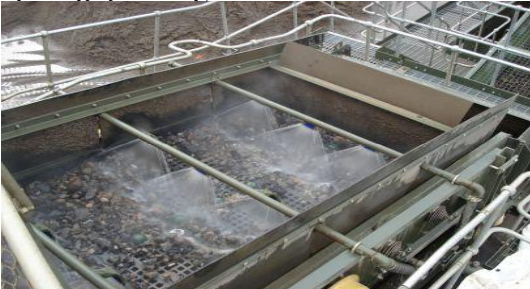
Fig 14 – Aggregate washing plant
