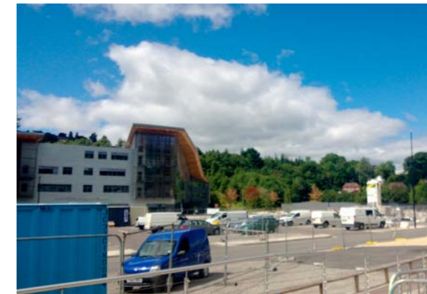
View west from adjacent to Network Rail land towards Learning Campus and future link (via a funicular) to Ebbw Vale town centre. Note works on site to create new public plaza. Proposed station will need to link into this plaza.
