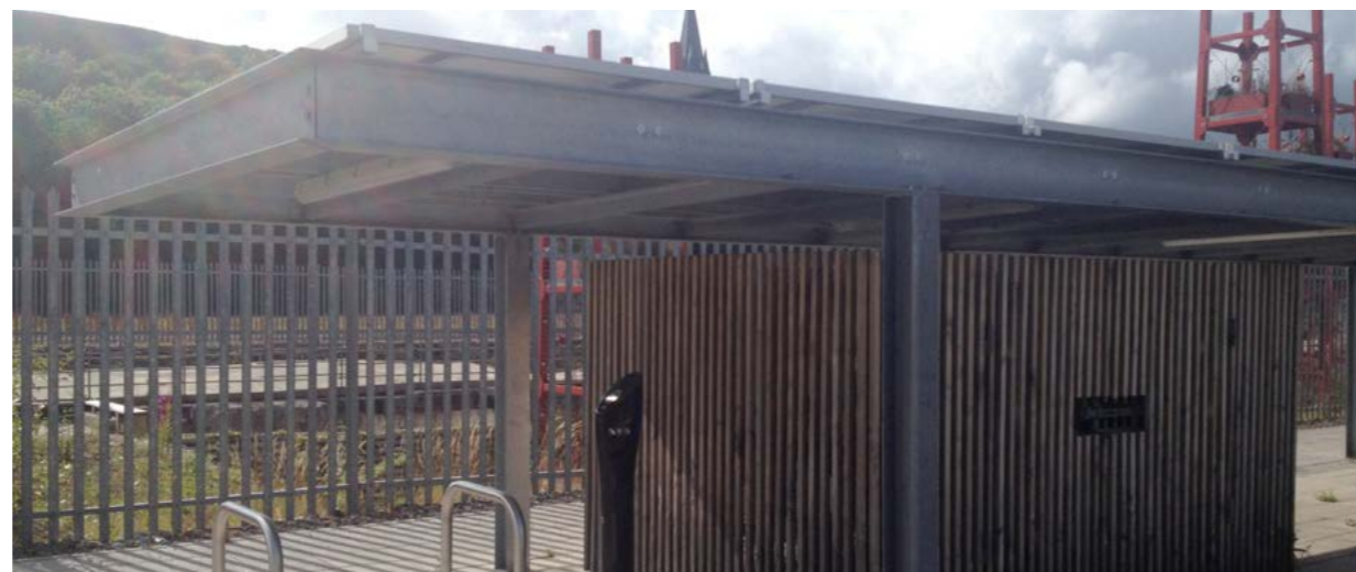
Galvanised steel structure
