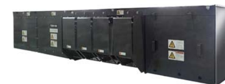
Auxiliary Power Unit with Dead Battery Starter
