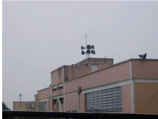
Photo 4.9: Sirens and rain meter in the remote alarm unit in the Morro da Formiga community. The equipment was installed on the terrace of a local school, also used as a temporary refuge in the event of extreme weather.
