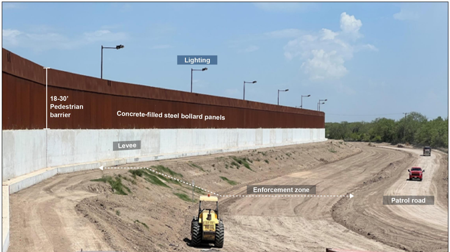
Figure 4: Border Wall System Program Components, Including Barrier atop a Levee, Rio Grande Valley, Texas (July 2022)
