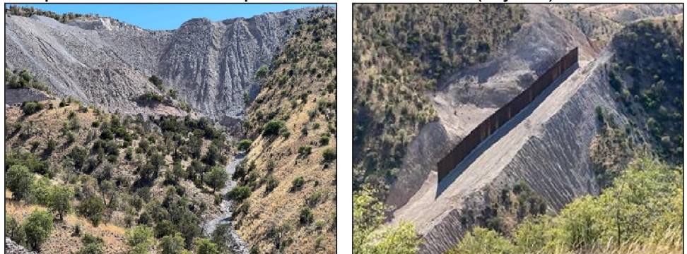
Erosion below the site of a cleared construction staging area (left); erosion below an area where only several border barrier panels were installed as of January 2021 (right).
