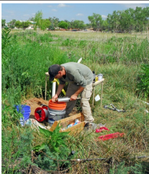
Figure 32. Constructing a groundwater monitoring piezometer at Blue Hole Ciénega in Santa Rosa.
