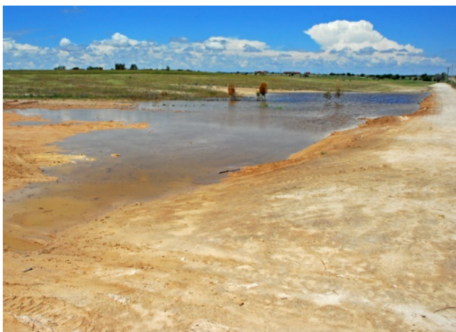
Figure 23. Diversion dike construction impounding and redirecting spring flow at Bass Lake ciénega in Santa Rosa.
