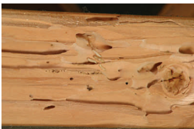
Drywood termite damage
