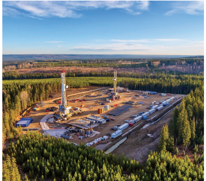
Above: Chevron is operating in the Duvernay shale formation near Fox Creek, Alberta, approximately 260 kilometers northwest of Edmonton, Alberta, applying best practices to reduce our operational footprint.
