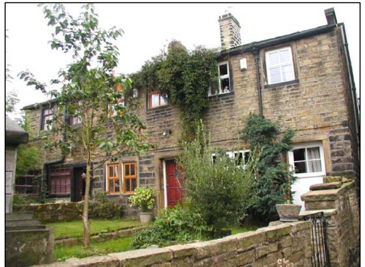
4-6 Hainworth are part of a cluster of buildings at the corner of Hainworth Lane and Hill Top Road. The range of window types and the painting of stonework undermine the unity of the group.
