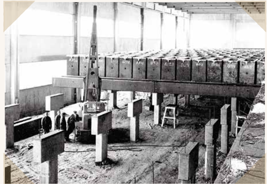
The cell house at Kokkola in the beginning of 1969. Production started in December the same year.
