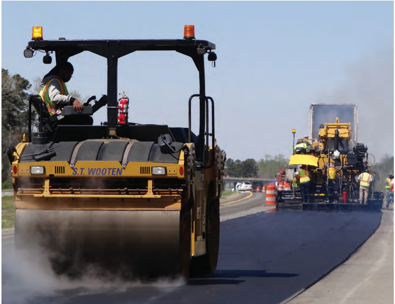
S.T. Wooten won a 2018 Green Quality in Construction Award for its repaving of I-795 in Wayne County, North Carolina. For the project, the company produced and placed more than 19,000 tons of an OGFC surface mix that included 5% RAS.
