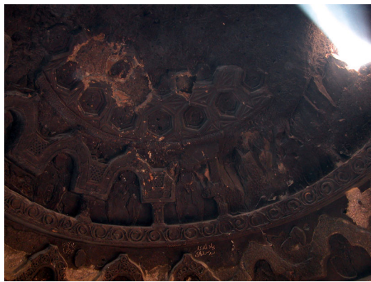
Figure 37: Bamiyân, grotto XI. Detail of the arcade's superior register and the cupola with sunken boxes. The gap through which light is filtering into the grotto is recent and is one of the signs the grotto is in danger of collapse.
