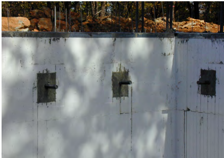
Figure 46 – Allowing the concrete to cure for at least 3 days before removing the OSB square pieces
