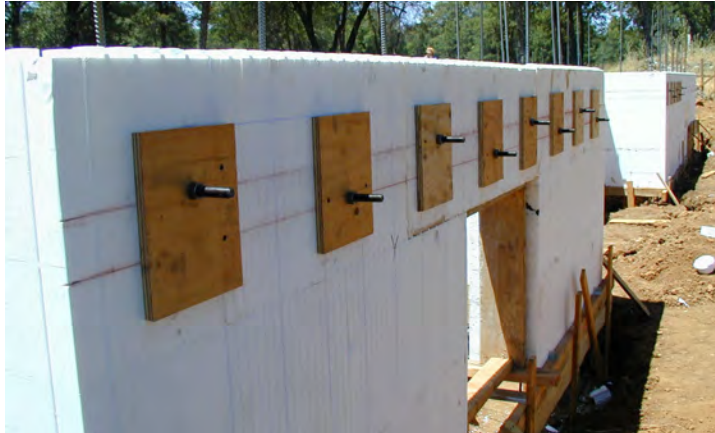
Figure 45 – Installing the OSB with anchor bolts onto the EPS openings and securing with drywall screws
