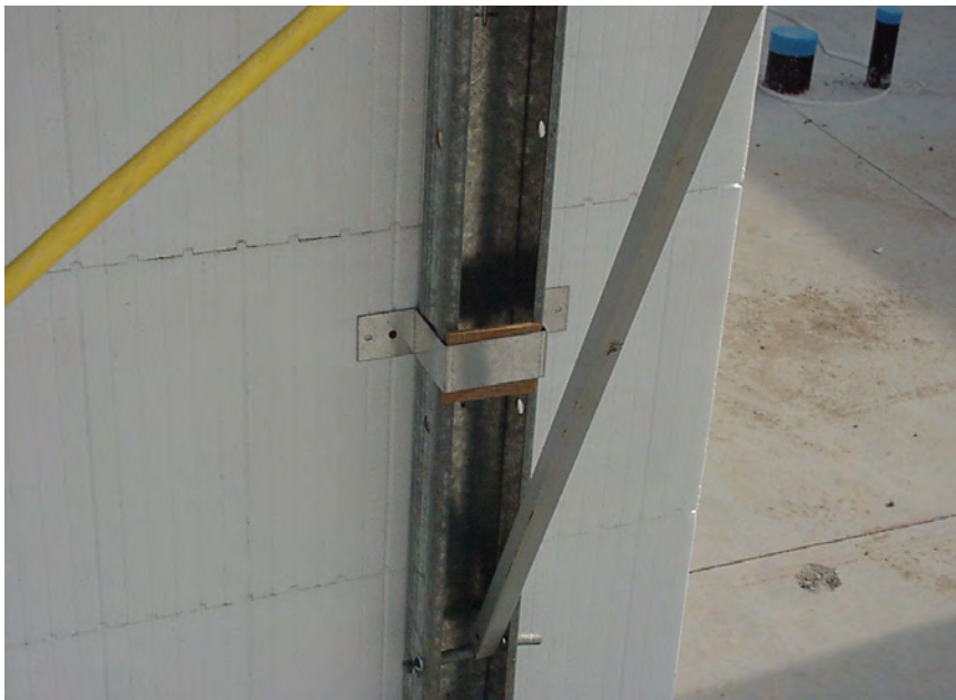
Figure 31 – A hat bracket wrapped around a vertical strong-back and screwed to webs on both sides
