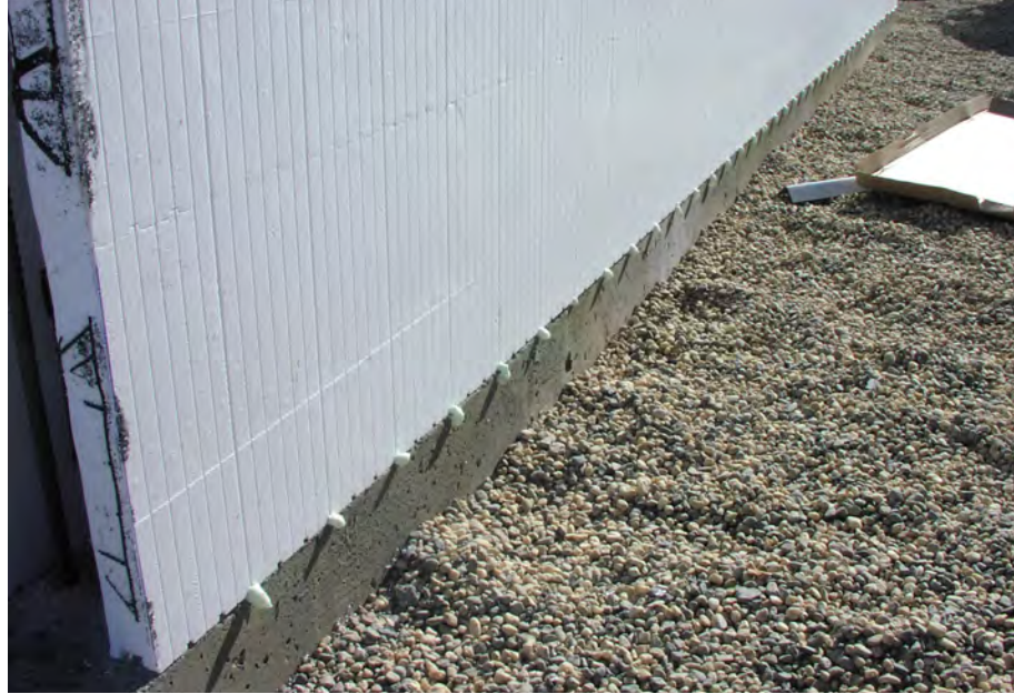
Figure 20 – Using foam adhesive to secure the first course of block to the foundation/slab
