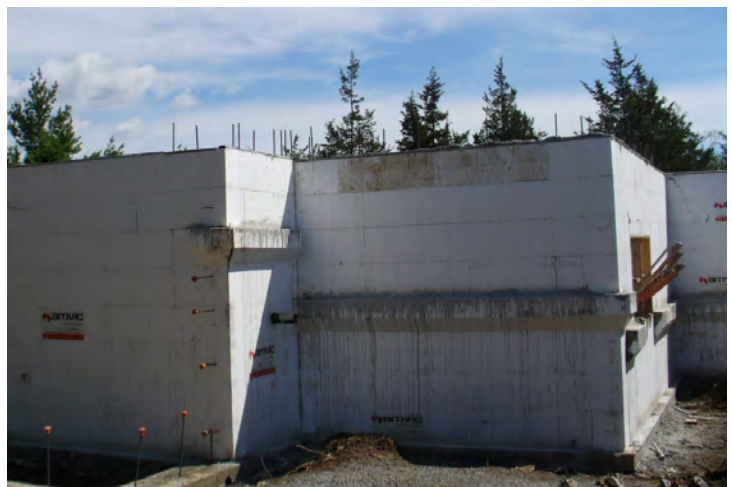
Figure 11 - Once the concrete had time to cure, remove bracing if not needed for following stages of construction
