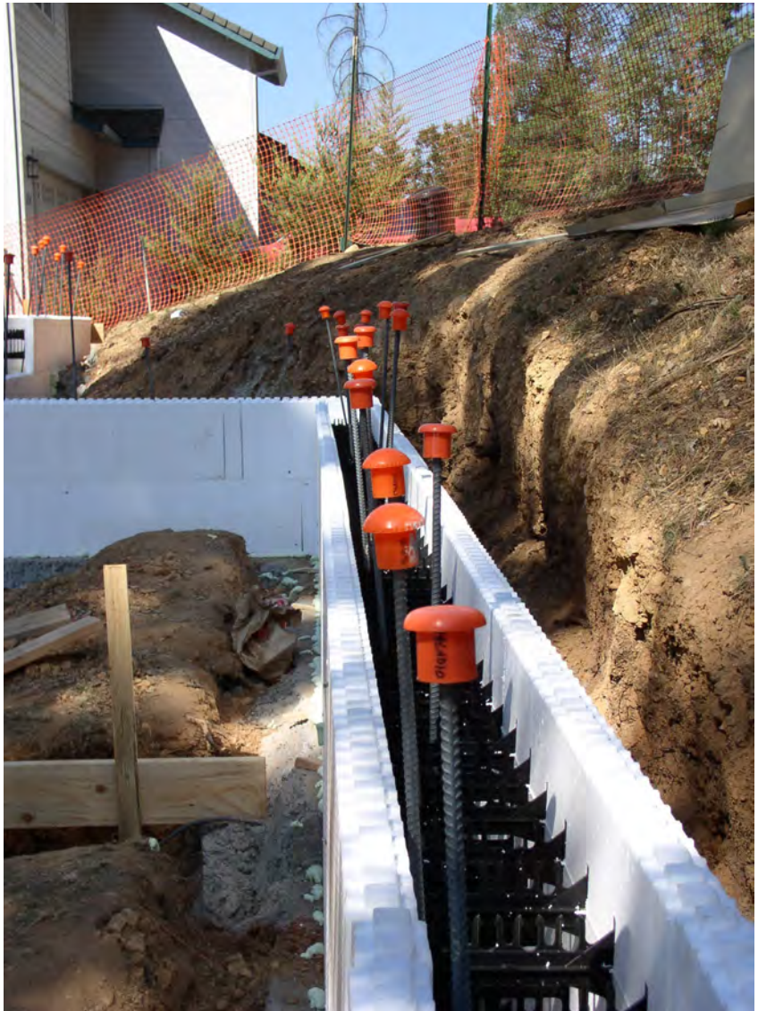
Figure 5 - Plastic mushroom caps on protruding steel bars
