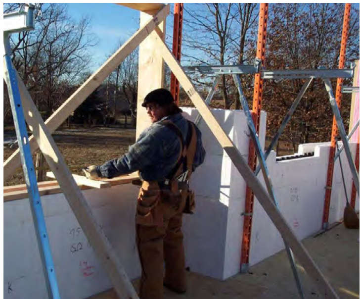
Figure 7 – Install alignment and bracing system around the interior of the perimeter wall
