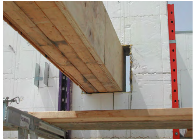
Figure 57 – Once the concrete is cured sufficiently, void fill is removed, and beam is installed
