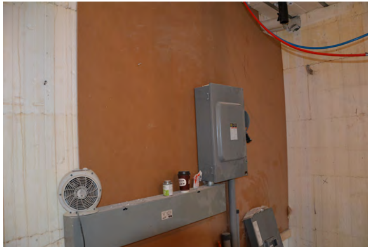
Figure 1 - Electrical panel installed on Amvic ICF
