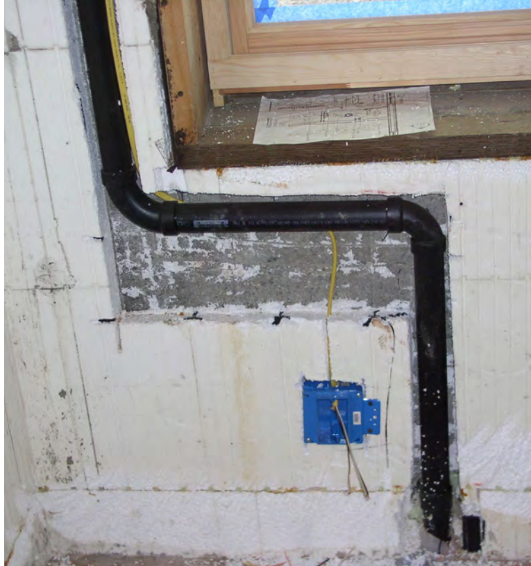
Figure 5 – Vent pipe embedded in the EPS foam
