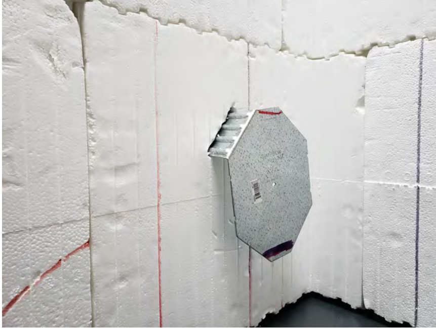
Figure 50 – Inserting the ICFVL long legs through the EPS and into the concrete
