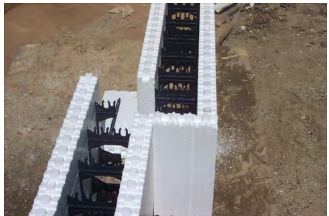
Figure 6 – Using cut off pieces to close the open ends and create a corner
