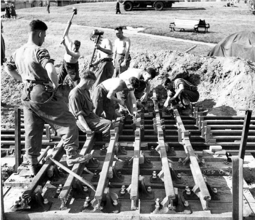
Figure 10: Pile mattress. The British emplaced their heavy (3.7 inch) guns on a solid base that became known as a “Pile mattress.” (Reprinted from Imperial War Museum.)
