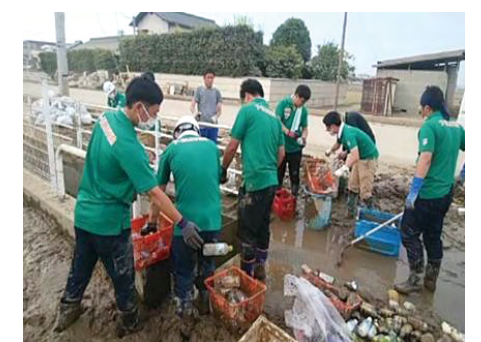
Restoration of a store inundated by the heavy rain event of July 2018
