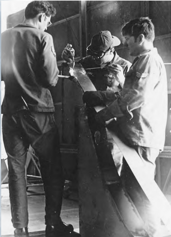
Tom Levesque, Ron Simms, and Leon Moores build hangar door inserts for the 1975 conversion of Building 254 for KC-135's. Also part of the team were Steve Hodgson, Gordon Ashburner, and Howard Towne.
