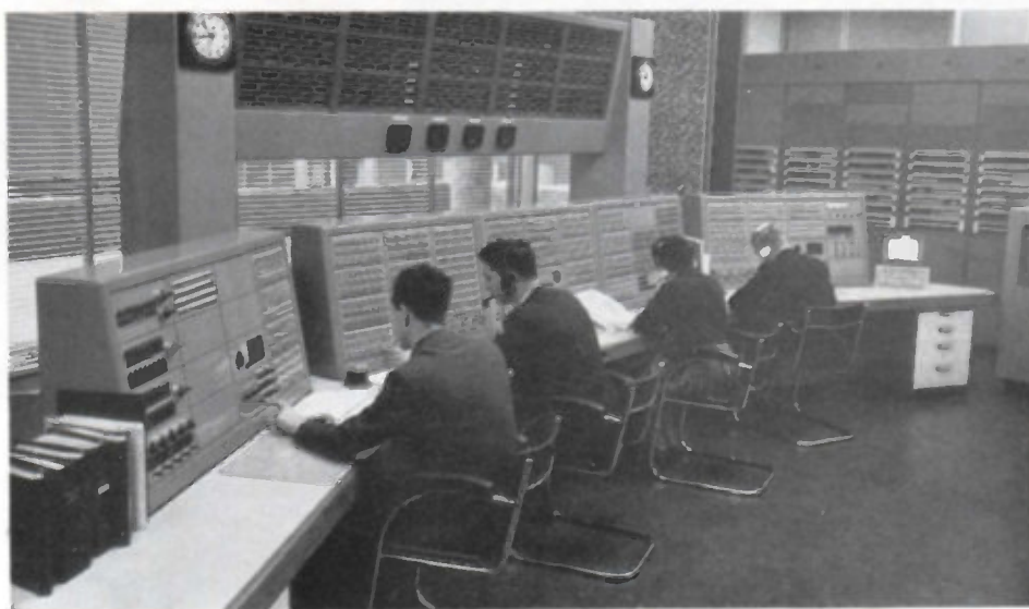
(below) The new Control Room in the Extension brought into operation in 1961. The main control desk shown includes facilities for the remote control of motorized selector switches by which any of 200 programme sources can be selected and connected to any of 130 destination lines. Over the desk is a large panel which indicates the source-to-destination connections in use
