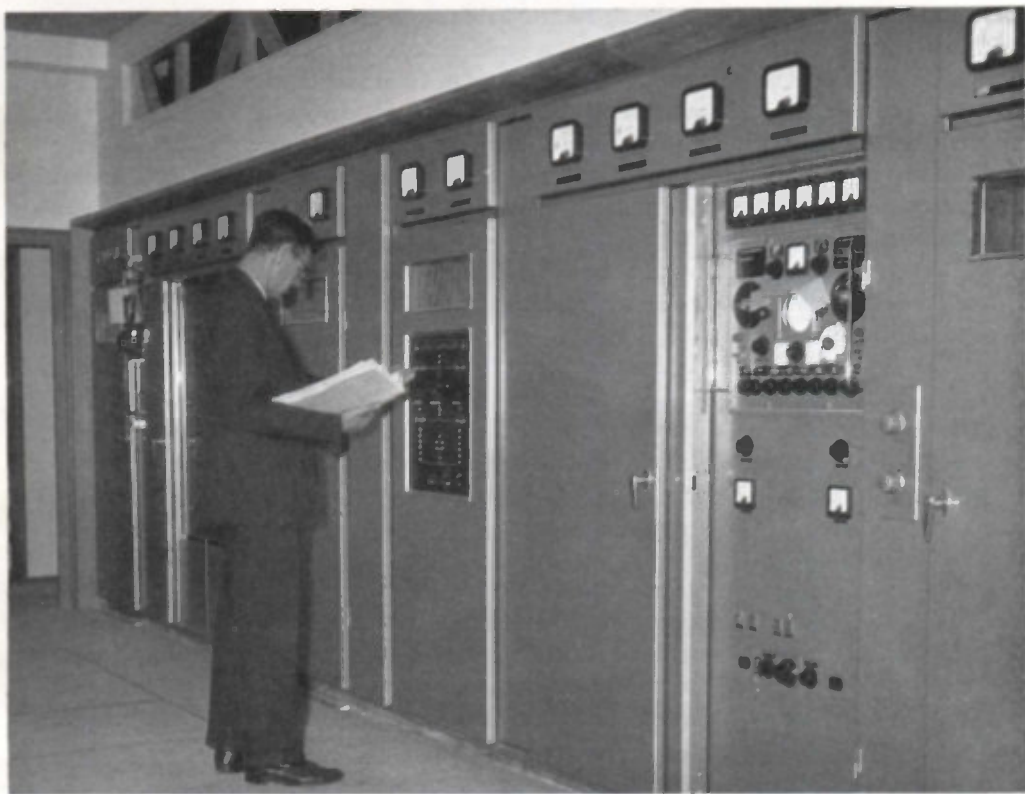
One of the two new 100-kW twin radio-frequency channel transmitters brought into service at Rampisham, Dorset, in 1961
