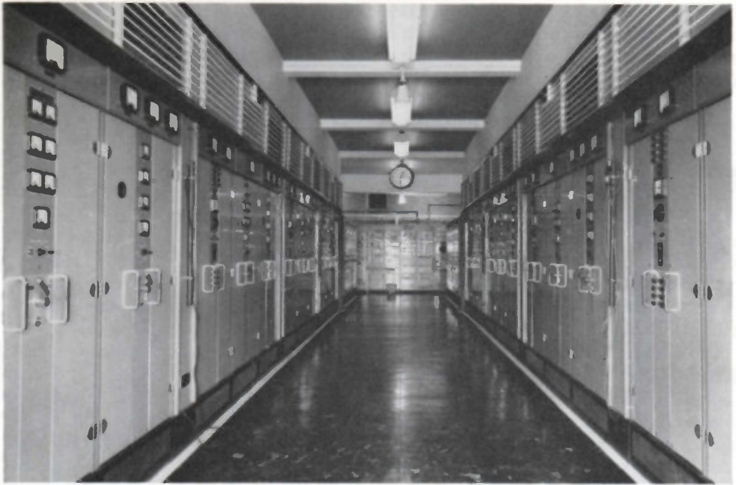
VHF sound station at Sandale, Cumberland: transmitter hall. This station radiates the North of England and the Scottish Home Services as well as the Light Programme and the Third Programme with Network Three. Each programme is radiated by a pair of transmitters, eight in all; four are shown on each side of the transmitter hall and beyond them are the programme input, drive, phasing, and automatic monitoring equipments. (Most VHF sound stations radiate three programmes and are therefore equipped with six transmitters)
