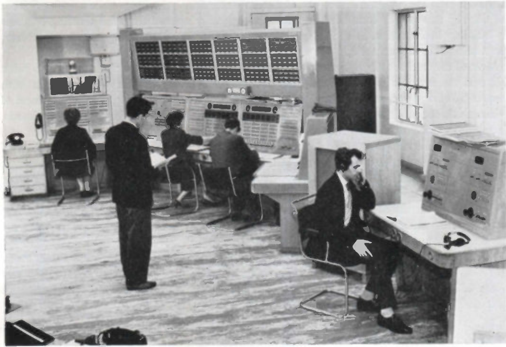
The Bush House Control Room. In the centre is the main operating position over which is the main source-to-channel indicator panel
