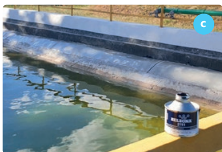
Photo 4. a) Repairs of damage to rubber and plastic elements, b) and c) sealing of expansion joints of fire prevention water tank
