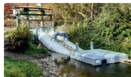
Fig. 5. Fishcon lock Leumühle at the river Aschacharm placed in the existing weir
