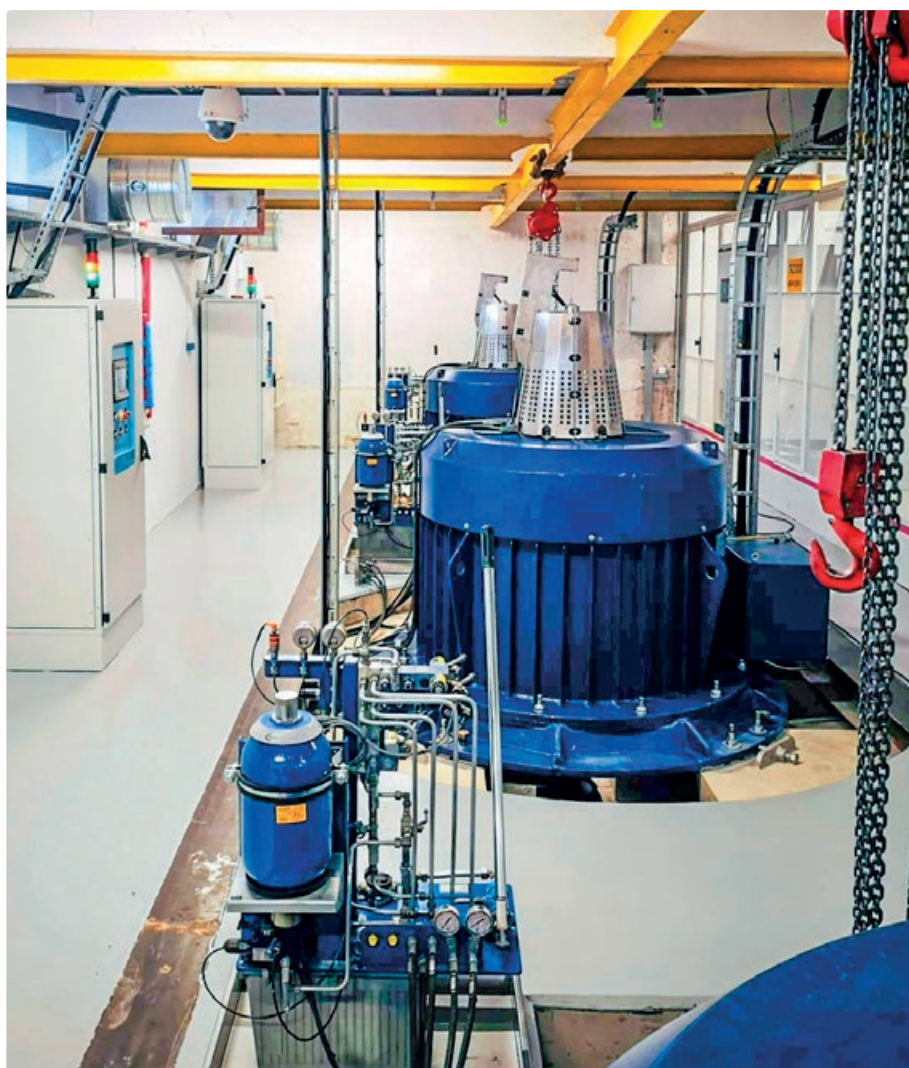
Fig. 7. Interior of the facility after repowering
