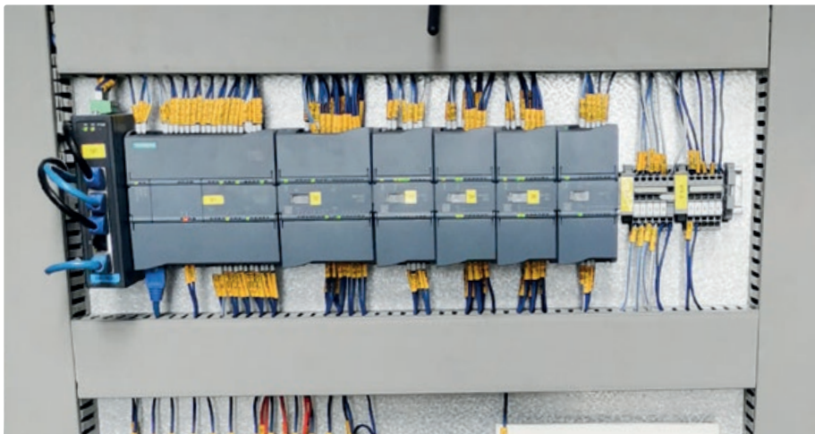
Fig. 6. View of the interior of control cabinets
