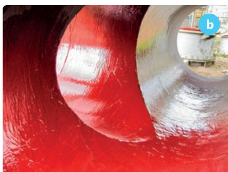
Photo 5. corrosion protection with BELZONA composite coatings: a) chemical storage tank, b) acidic fume outlet duct
