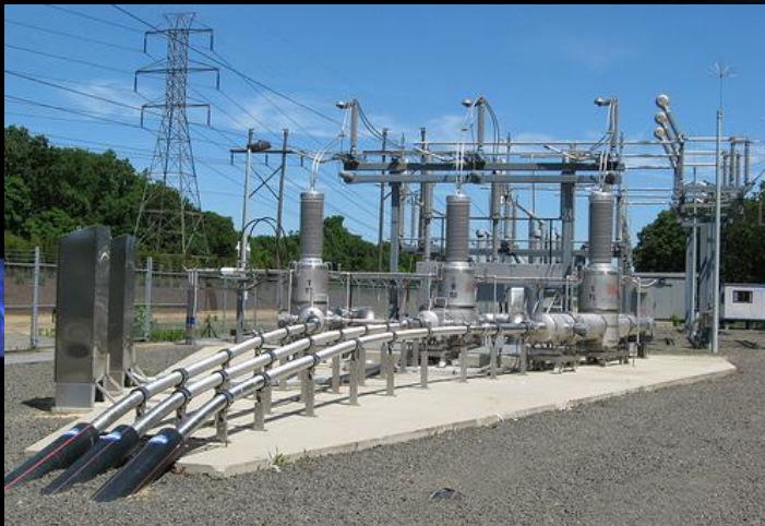
Underground transmission lines
