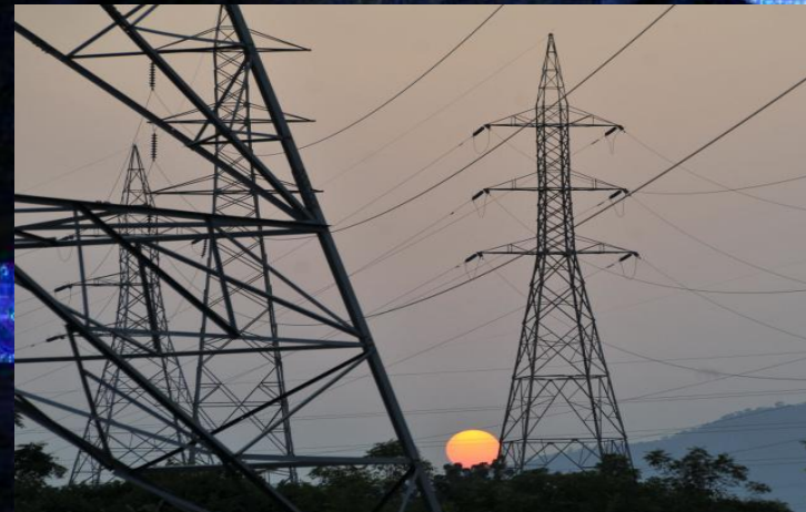
Overhead transmission lines
