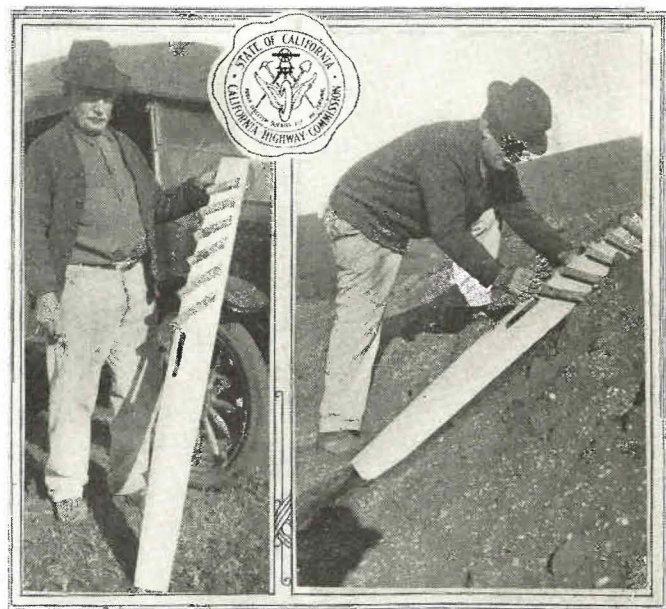
ON THE MALIBU JOB —A straightedge with cleats at various angles used for checking slopes on the Malibu Ranch grading contract, Division VII. This device was described in the December issue of the Bulletin.
