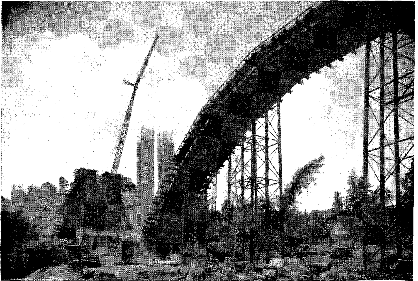
Upper—Observation post for sidewalk superintendents on site of Colorado Freeway bridge in Pasadena. This building erected by Guy F. Atkinson Co., the contractor. Lower—Construction operations on Colorado Freeway bridge as viewed from observation post building.
