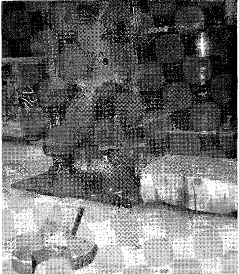
Detail showing 2-inch screw jacks which have been partially lowered. 100-ton hydraulic jack at right carried column load while screw jacks were being lowered. Grout pads which had been placed between the column bases and the concrete footings during concrete placing operations have been removed.
