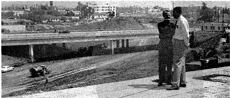
Looking southeasterly from roof of KTTV studio along Hollywood Freeway showing construction in progress. Wilton Place overcrossing in foreground. Roy Maypole, KTTV producer, left, interviews Haig Ayanian, Resident Engineer, Division of Highways, during broadcast of Sidewalk Superintendent television program.
