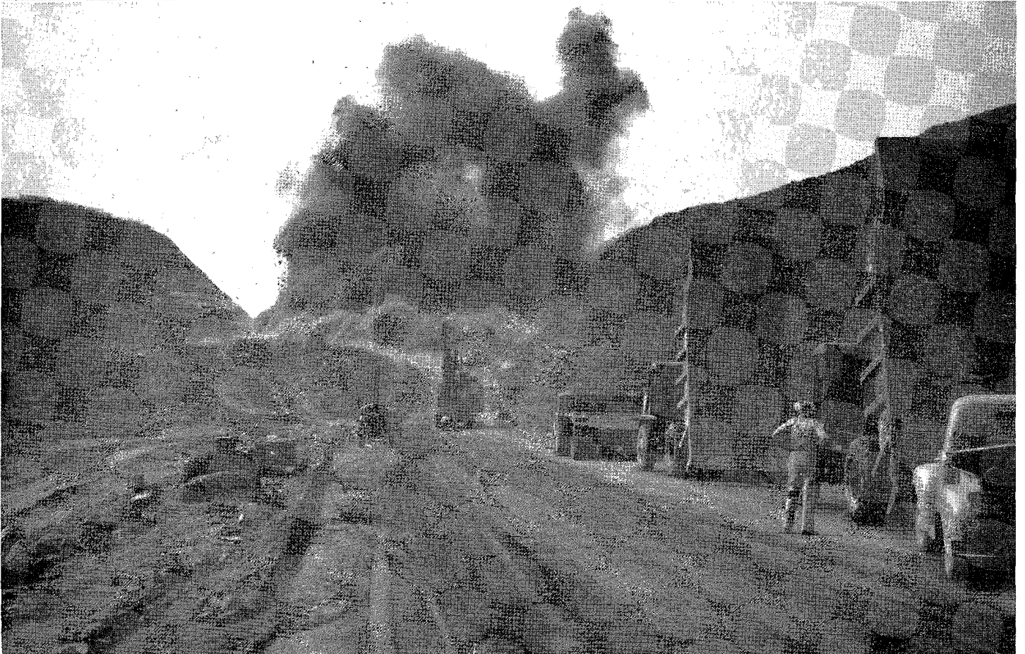
Upper—La Cadena freeway section of U. S. 395 between Riverside and Colton, constructed in 1950. Lower—Blasting the big cut on the unit of U. S. 395 currently under construction between Antelope Road and State Sign Route 74.
