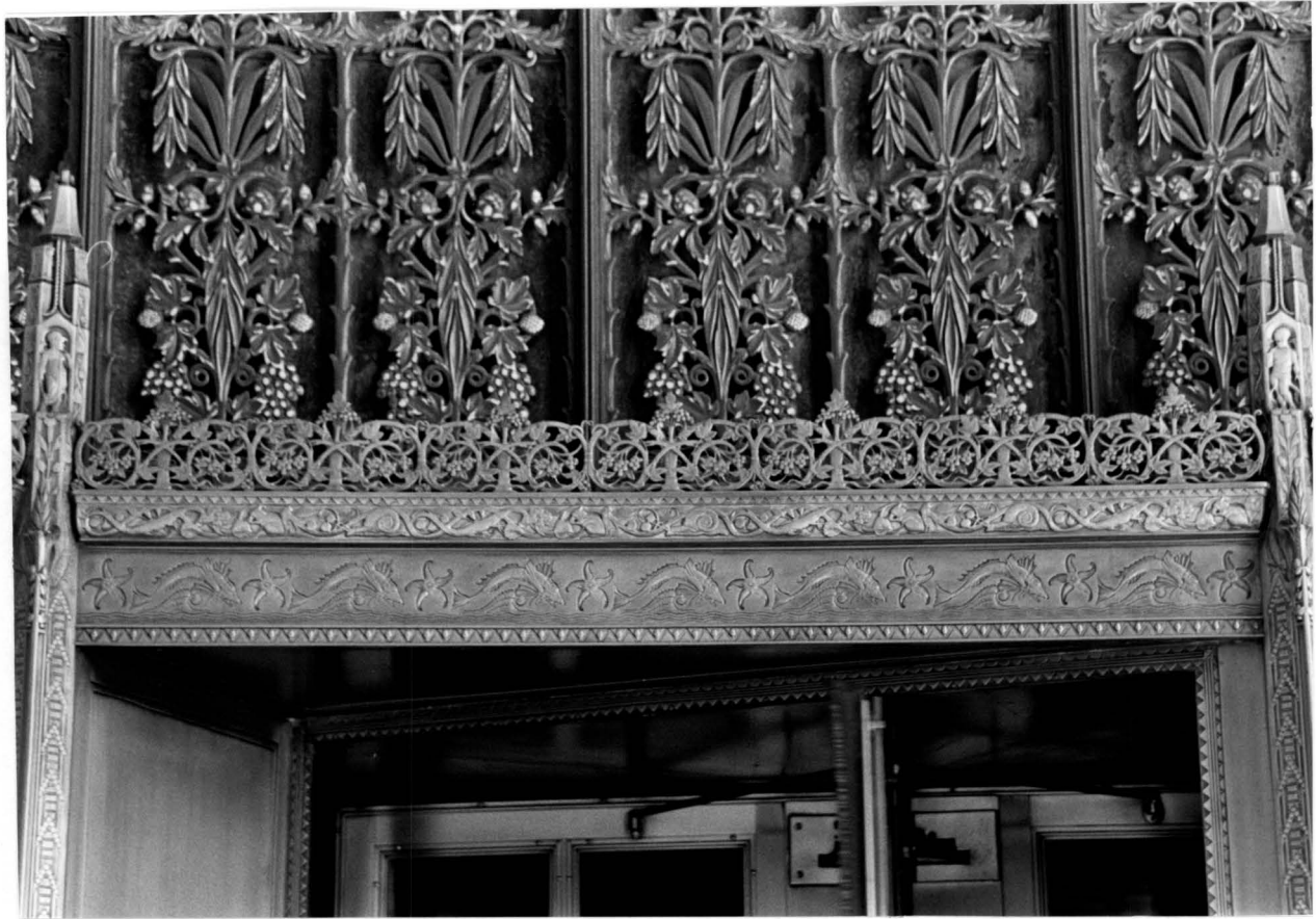
Fig. 8: Entrance detail showing top of door frame and lower part of bronze window grille. (Photo Credit: Carl Forster.)
