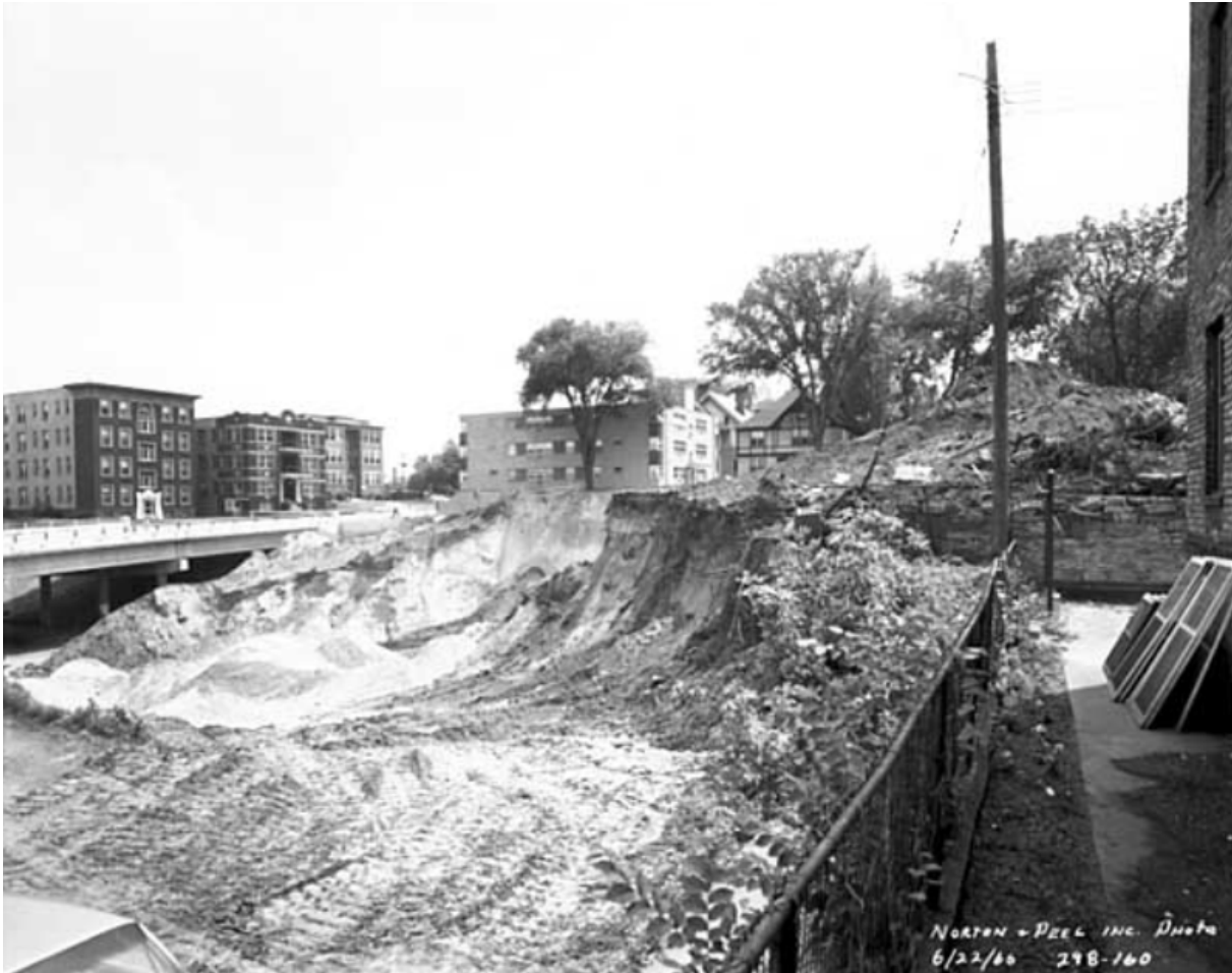
Construction of Interstate 94 looking towards Blaisdell Avenue in Minneapolis, June 22, 1966. Norton & Peel Photograph Collection, Minnesota Historical Society.
