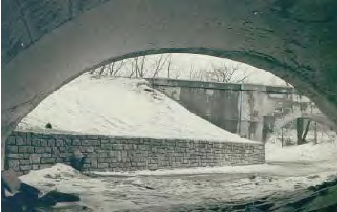
Figure 2.6 Retaining walls along Minnehaha Creek were constructed by the WPA and are characteristic of the types of infrastructure projects that the WPA constructed throughout Minneapolis and the country at large. Retaining walls along Minnehaha Creek, c. 1938. Walter B. Dahlberg, The Story of W.P.A. in the Minneapolis Parks, Parkways, and Playgrounds for 1938 ([Minneapolis, MN?]: Board of Park Commissioners, 1939).
