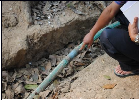
Photo 10: Gas pipe joints/ butt joint
