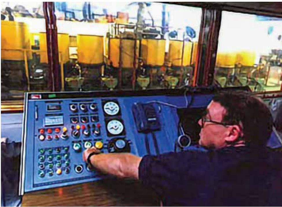
Figure 4. SCAMP loader from control room.
