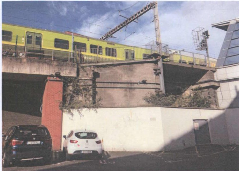
9. View of screen wall below viaduct extension to front of smaller vaults.
