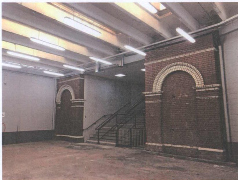
6. View of blind arches either side of granite steps from former station hall.
