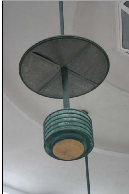
Sunset Play Center Bath House, First Floor Interior Detail of hanging lamp Photo: Carl Forster
