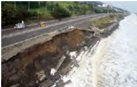
Figure: Seawall damaged by a typhoon
