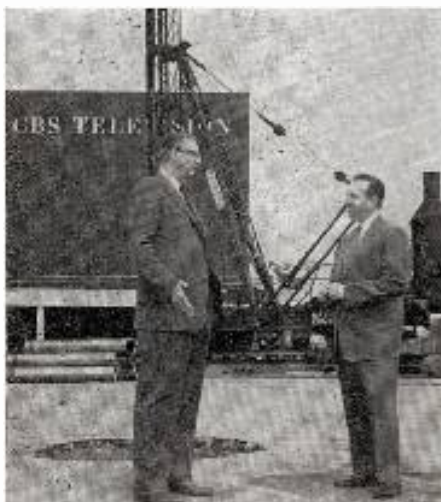
ON-SITE inspectors as work gets underway on expansion of CBS-TV's Hollywood Television City are Howard Meighan (l), vice president in charge of the Western Div., and Frank Michal of the network's Production Services Div.
